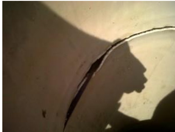
Photo 3. Example of unsuitable adhesive cause of delamination (Dan Chamberland, 2014)
