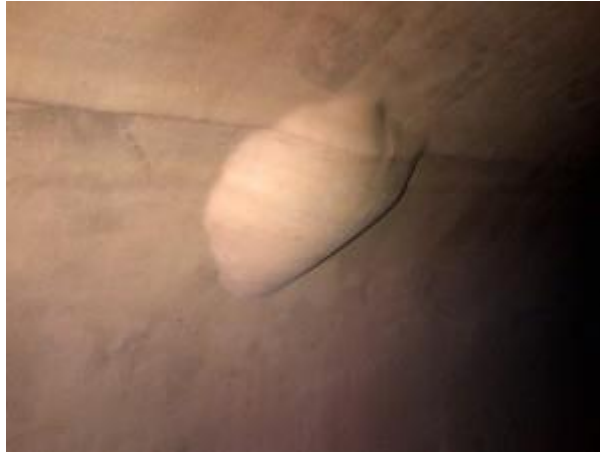
Photo 5. Bubbling due to misapplication (Dan Chamberland, 2014)
