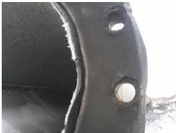
Photo 2. Delamination at the edges (Dan Chamberland, 2014)
