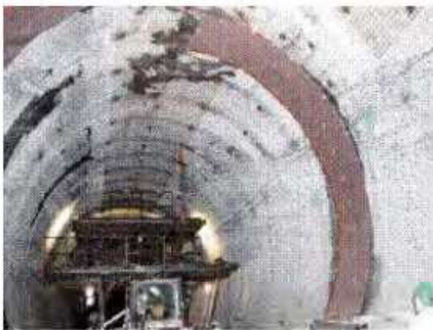
Figure 22. 120.000 m 2 of DELTA®-MS with a flame retardant quality were integrated in the tunnel of Chatahouchee.
