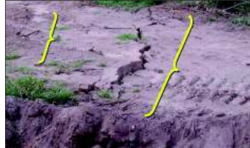
Figure 2: Cracks of decompression in header of slope mining
