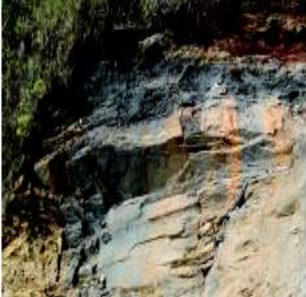
Figure 5: Toppling block in the slope at Vila Aparecida neighborhood.
