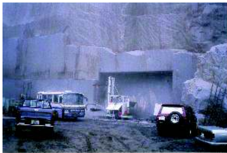
Figure 1. Tunnel excavation in a Japanese quarry by means of waterjet slotting equipment
