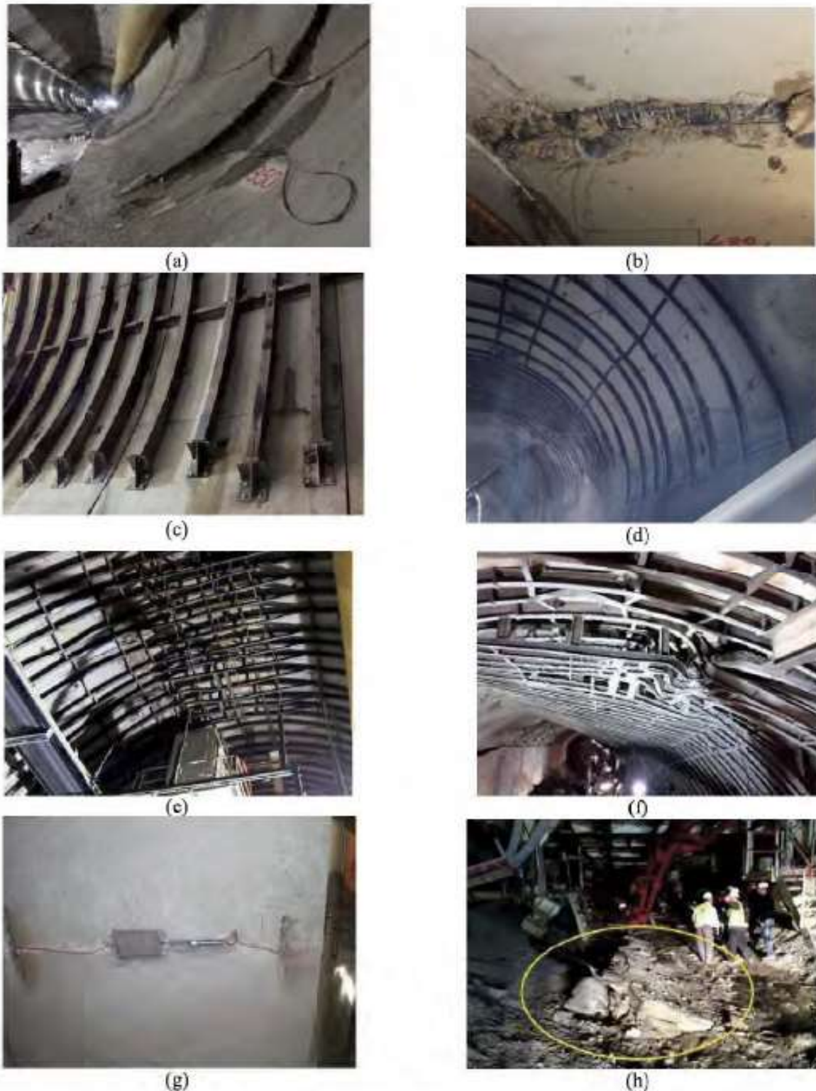
Figure 2. a) Observed some damages in the segmental linings b) A damaged segment in the crown c) Steel beam haunches d) Additional steel-beam with wire mesh and fiber reinforcement shotcrete support e) Steel framework in the crown f) Plastic deformations of I-beams g) A segment with the load monitoring devices h) Segment failures in the tunnel invert
