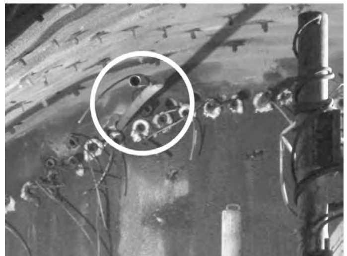
Figure 6: Broken pipe because of a collapsed pre-drilled hole at the Trojane tunnel
