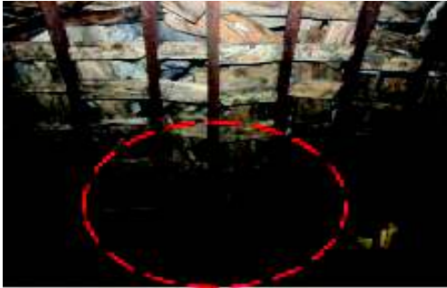
Fig. 11 Deformation on steel supports
