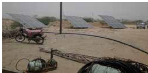
Fig. 6. Solar panels producing electricity for pumping stations.
