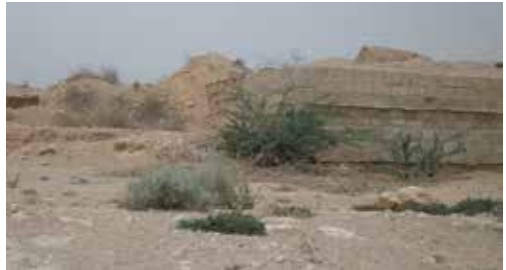
Fig. 5. Showing collapsing of Malir River banks
