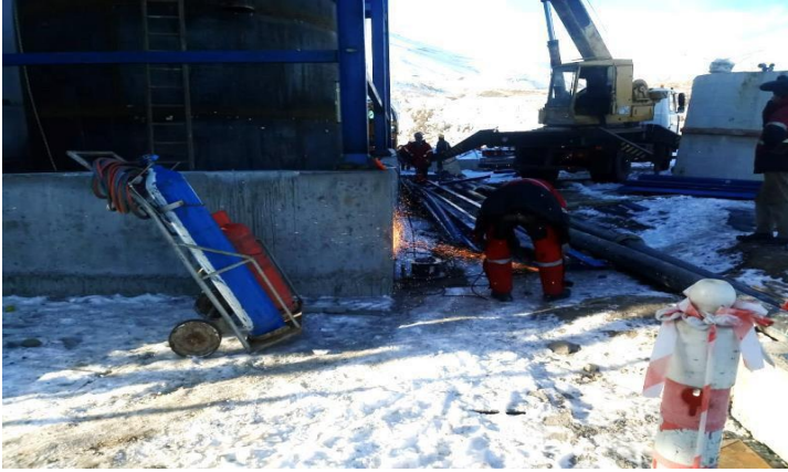
Figure 2. Dangerous situation during the welding process
