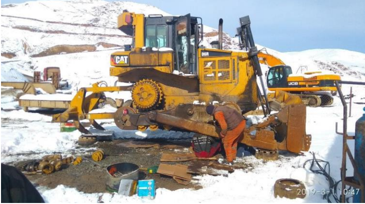
Figure 6. The dangerous situation occurred during the fixation of dozers
