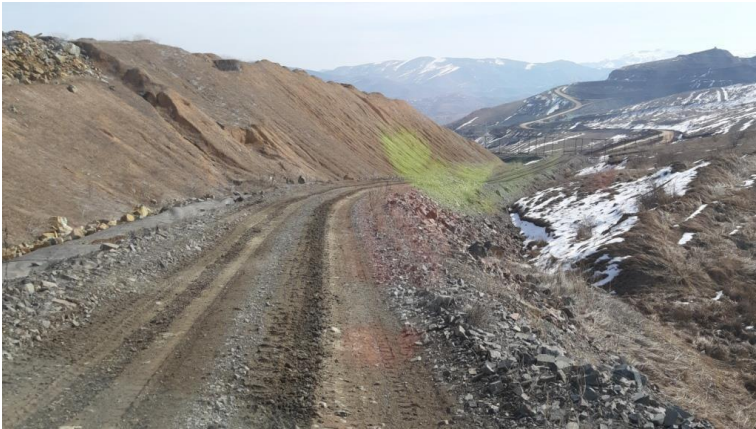
Figure 7. The dangerous situation occurred in the road
