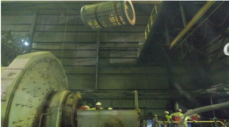
Figure 11. The dangerous situation due to the lifting operations.
