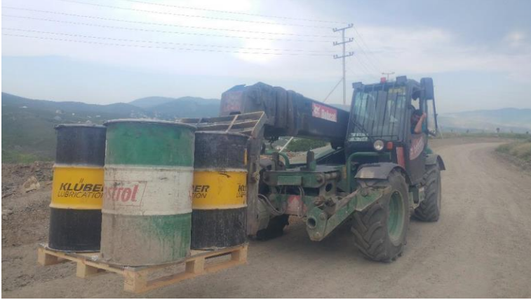
Figure 8. The dangerous carrying of the drums by telehandler.
