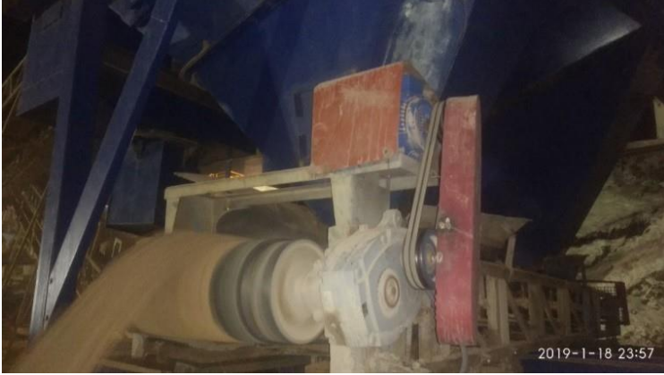
Figure 4. The photograph showing the dangerous situation occurred during the working of conveyor system
