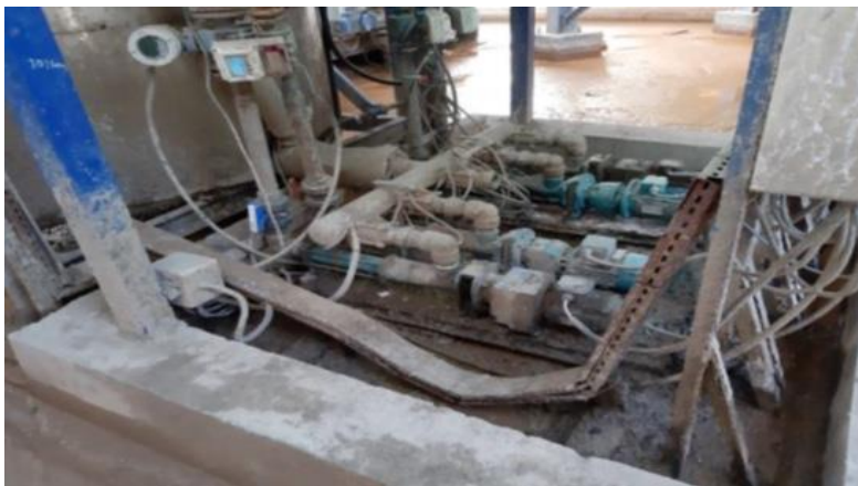
Figure 1. The photograph of electrical cabling
