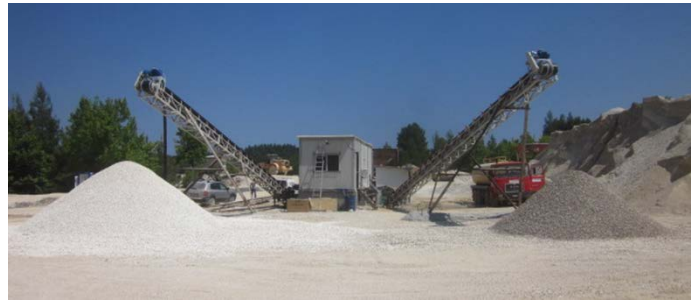
Figure 4 Example for sorting plant
