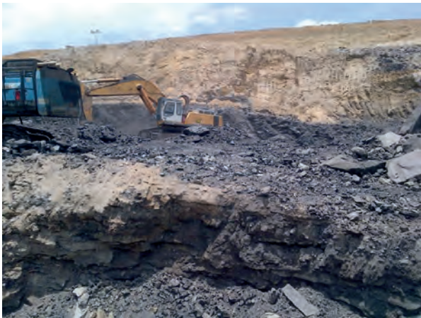
Figure 10. An excavator that has underwent breakdown
