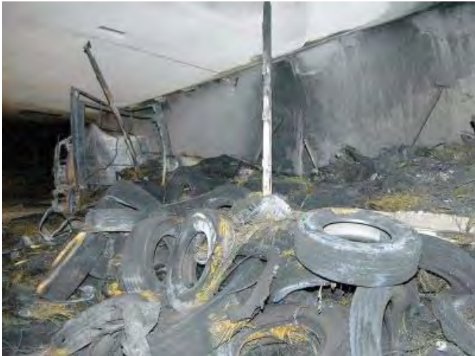
Figure 3. Fire accident in the Fréjus Tunnel (France) on 4.6.2005.
