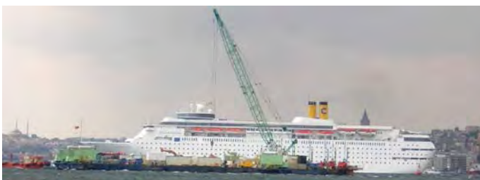
Figure 17. Views of dredging work and passing international and domestic ships nearby the construction site
