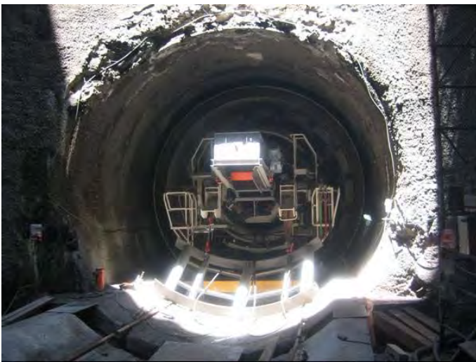
Figure 9. TBM pushed forward for gantry placement with the help of steel pushing frames
