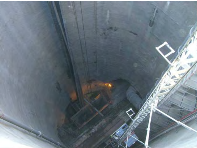
Figure 17. Vertical conveyor band as seen from the top of the shaft
