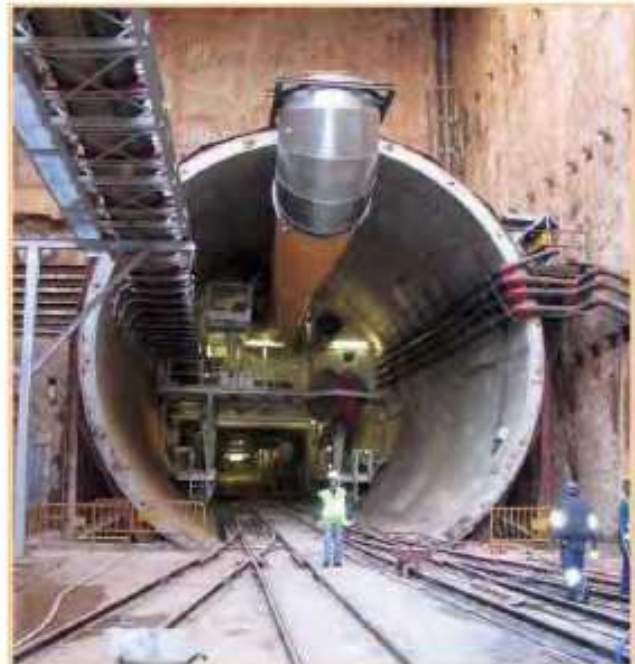
Figure 1. Barcelona metro line 9: monitoring of hydro-geological parameters and of the existing infrastructure during the construction of 43 new stations of new line in soft soils
