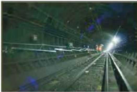
Figure 10. Chain of electrolevel sensors to monitor the longitudinal deformation of a tunnel
