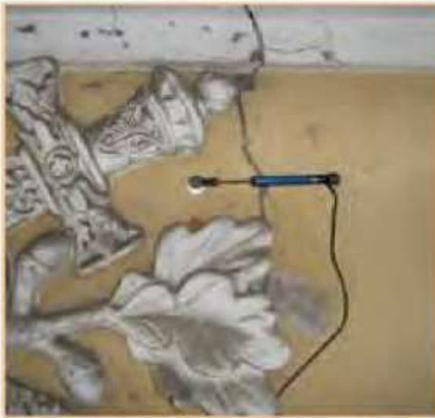
Figure 12. Crack meter performing continuous measurements of the crack opening
