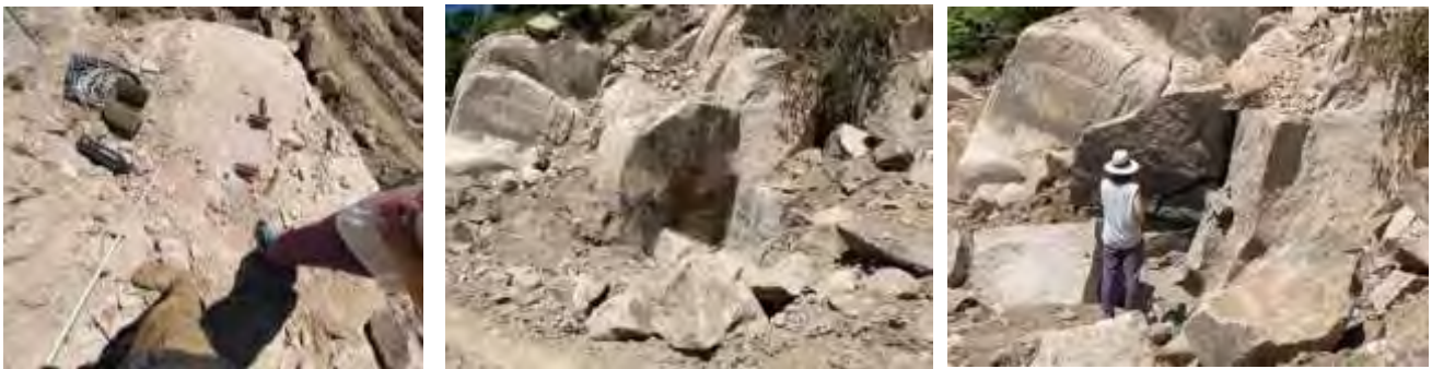
Figure 8. Splitting of rock body with two parallel boreholes. Effects from preloaded bottom charge of 300 g. Mixture #3 and decked second charge of 150 g. Mixture #3 in every single blasthole with length 1,80 m.
