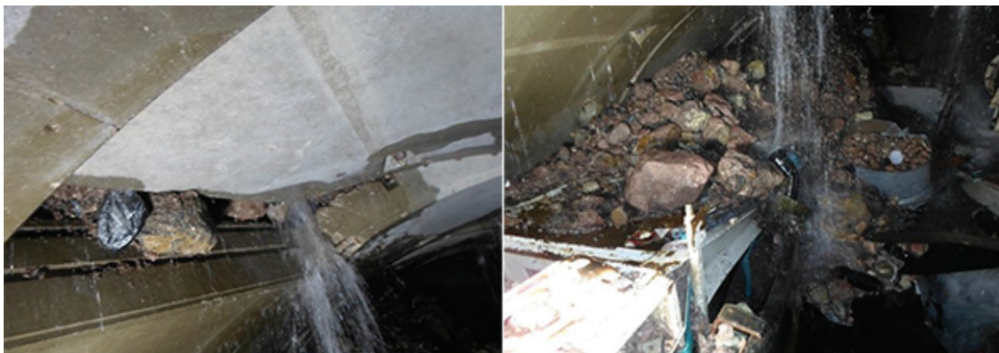
Figure 5 Failure of segments in Gerede Tunnel
