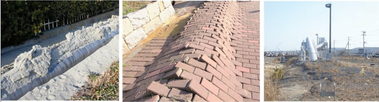
Figure 4. Examples of uplifted underground structures in liquefied ground
