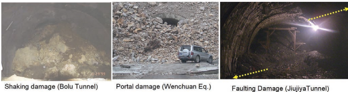
Figure 3. Examples of earthquake-induced damage to underground structures.
