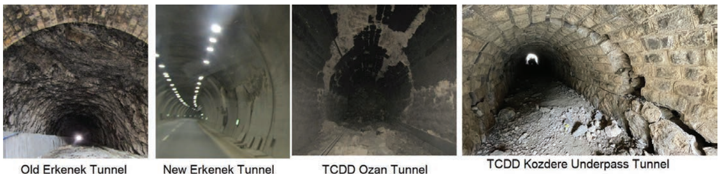
Figure 21. Views of damage to roadway, railway and underpass tunnels caused by the Pazarcık earthquake.
