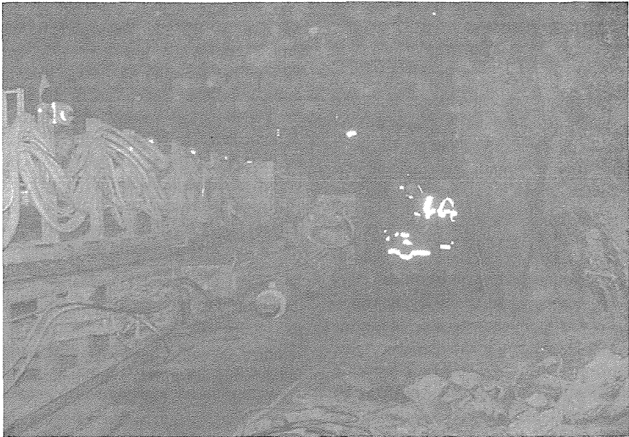
Figure 3. Showing the DMU propulsion cylinders and roadway which the FCT sits on.
